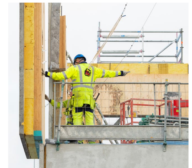
Hybrid elements are being used in the construction of Metsä Fibre's Rauma sawmill.
